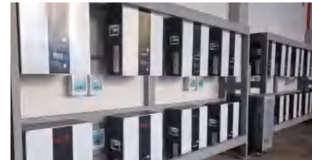
Wall-mounted lithium battery
